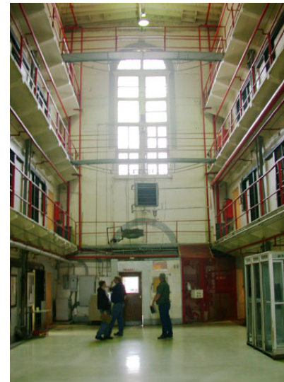
Views of Main Corridor with Unit Heaters
