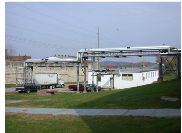
Overhead Steam, Condensate & DHW Piping from Boiler Plant
