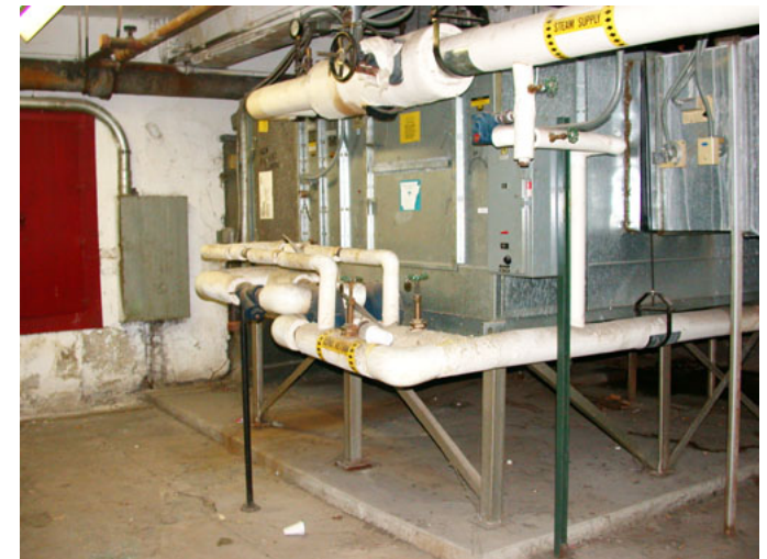
Basement Heating and Ventilating Units
