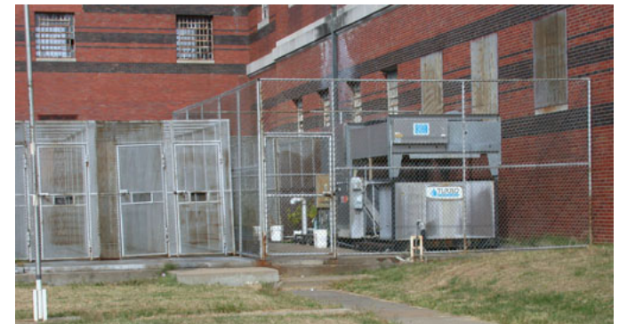
Ice Plant Equipment
