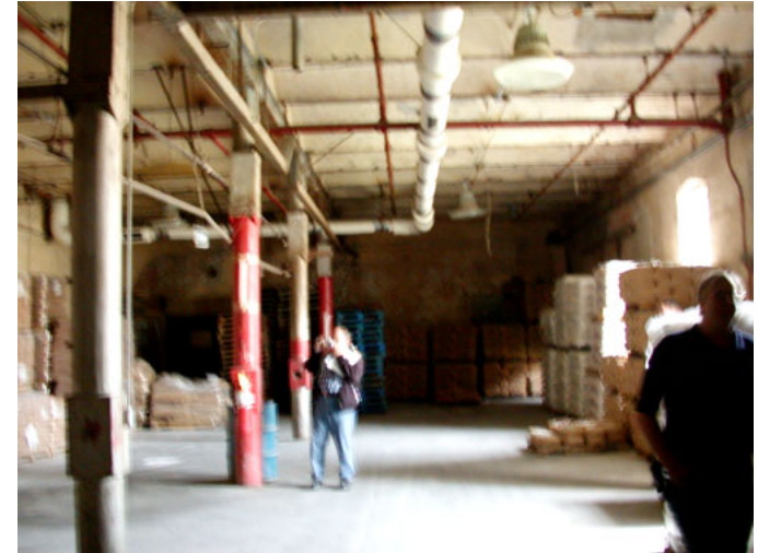
Basement Storage Room – Steam Pipe
