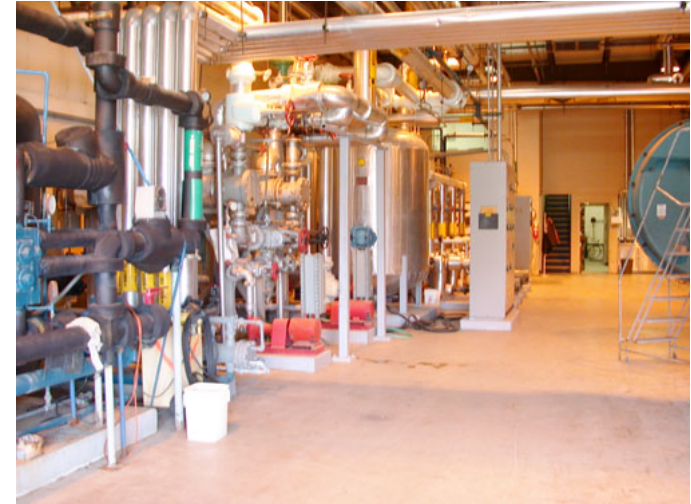
Boiler Plant Auxiliaries
